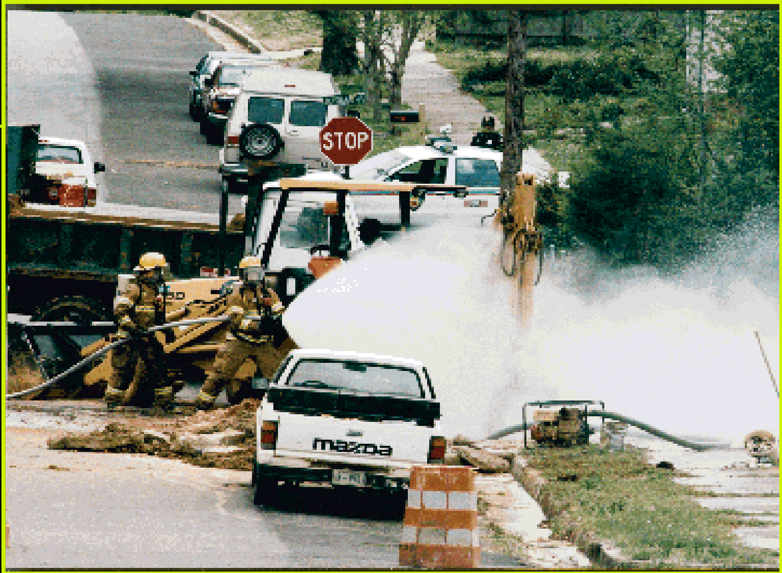
Gas Main Rupture: Firefighters provide water shield to prevent explosion
